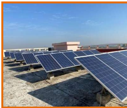
10 KVA Solar Panels fitted at Roof Top of the College Building
